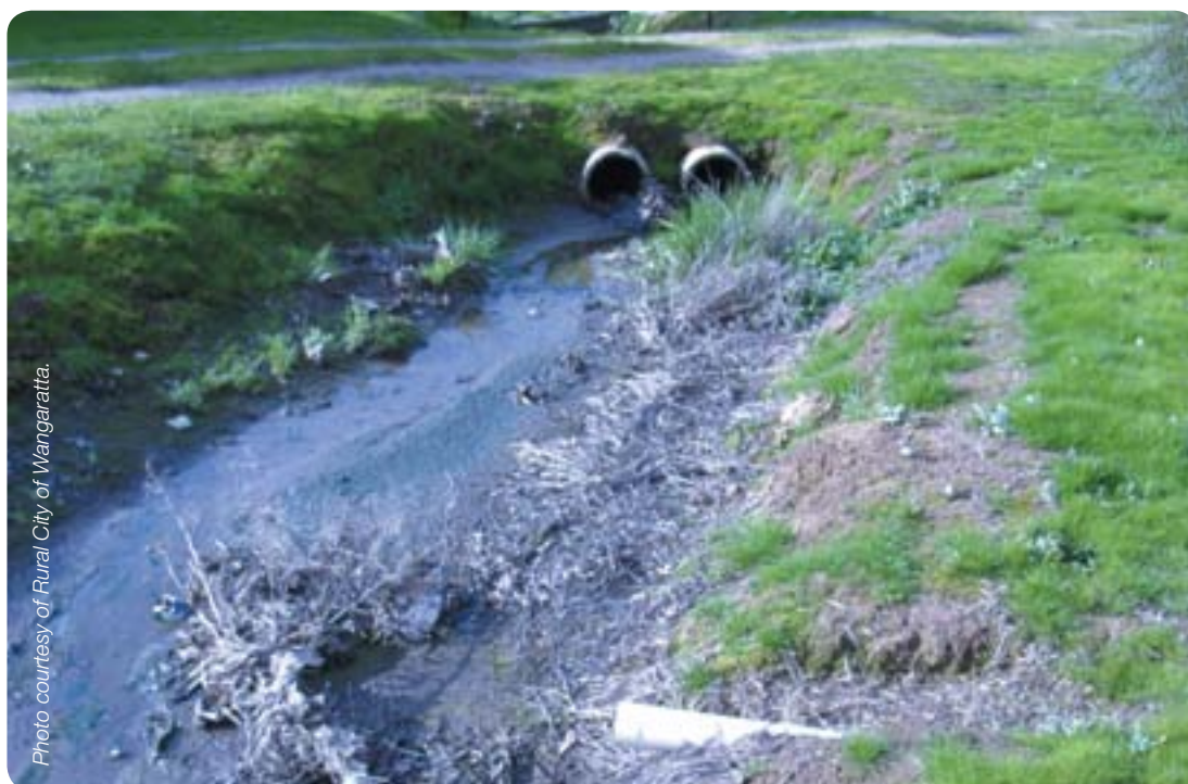
Waste that is disposed of inappropriately can enter raw water supplies via stormwater drains.
